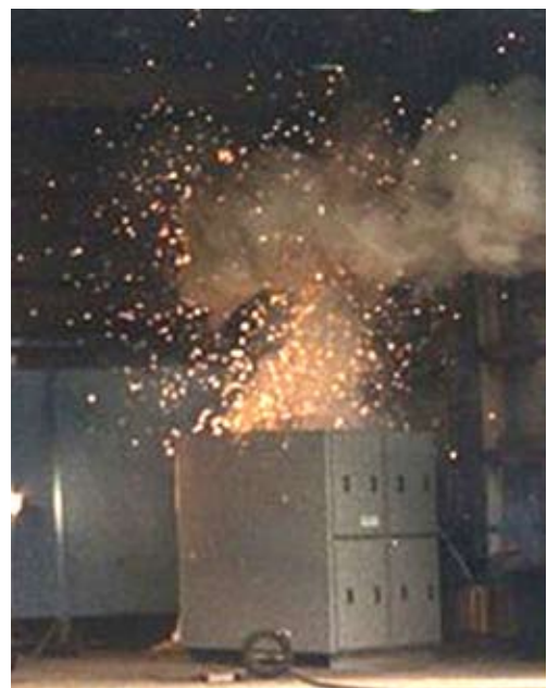
AN ARC FAULT IS A VERY DESTRUCTIVE FORCE
