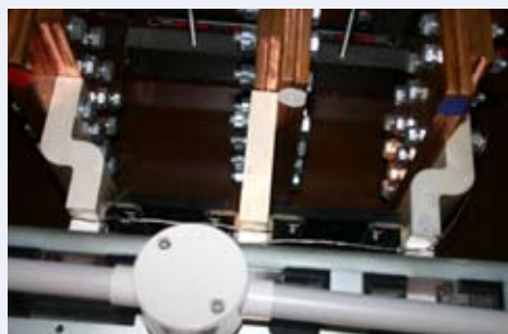
ARC INITIATING FUSE WIRE ON ACB MAIN TERMINALS
