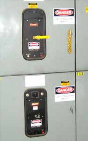
Obsolete main circuit breaker
