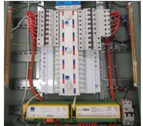
Panelboard fitted with RTS
