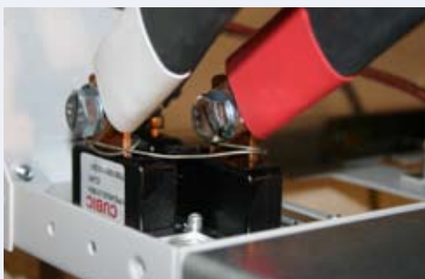
ARC INITIATING FUSE WIRE WRAPPED AROUND BUSBAR CONNECTION PIECE
