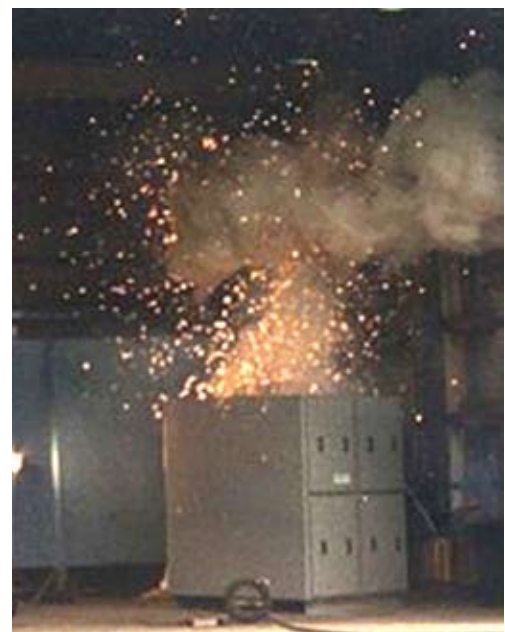
AN ARC FAULT IS A VERY DESTRUCTIVE FORCE
