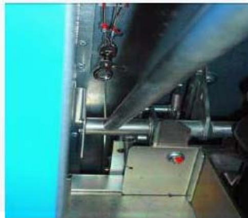
Photo 11: Operating handle in drilling space
