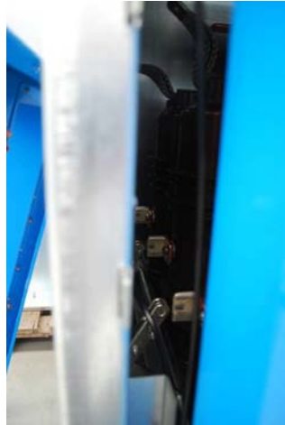
Photo 15: Earthing knife arc-killer is moved out of the earthing block
