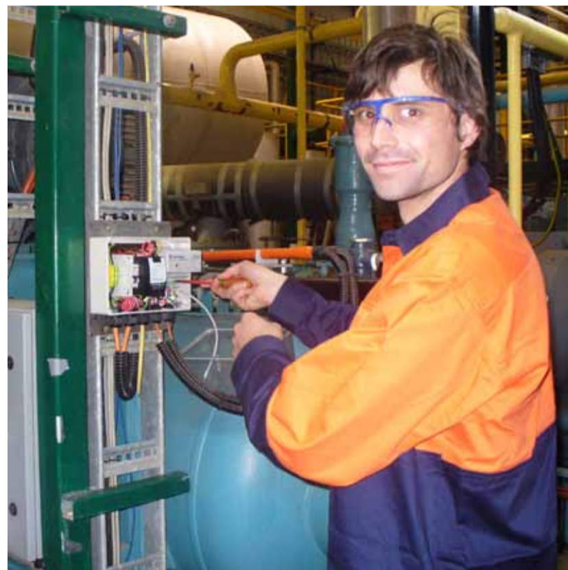
(above) Lenny Guetlich from the Fletchers International WA Electrical Department working on the CBM installation.
