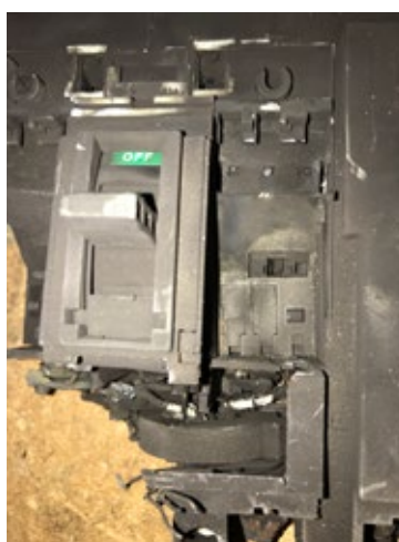
Notice, breakers is “TRIP” position, however contact welding can cause arc fault currents to continue to flow in the circuit.
